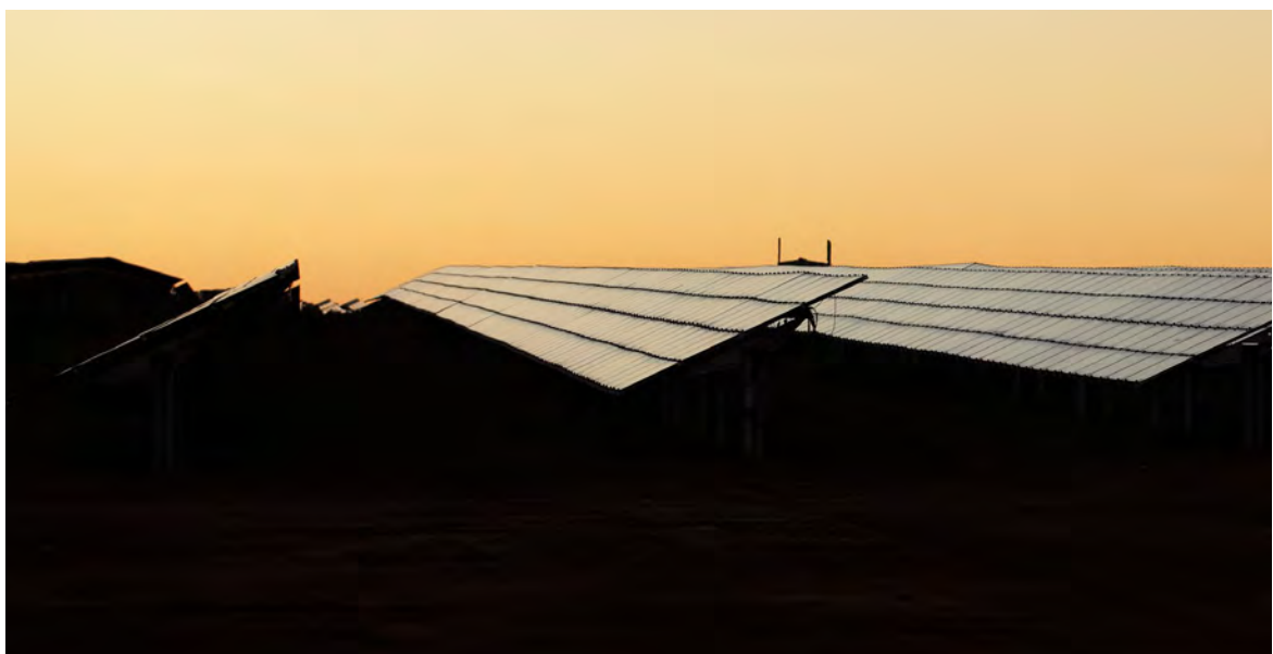
Above image: Broken Hill Solar Plant
